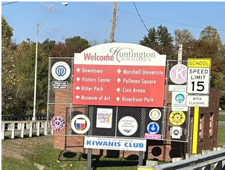
Rewrapping the existing welcome signage on Hal Greer Blvd. next to Meadows Elementary. 140 inches x 96 inches
